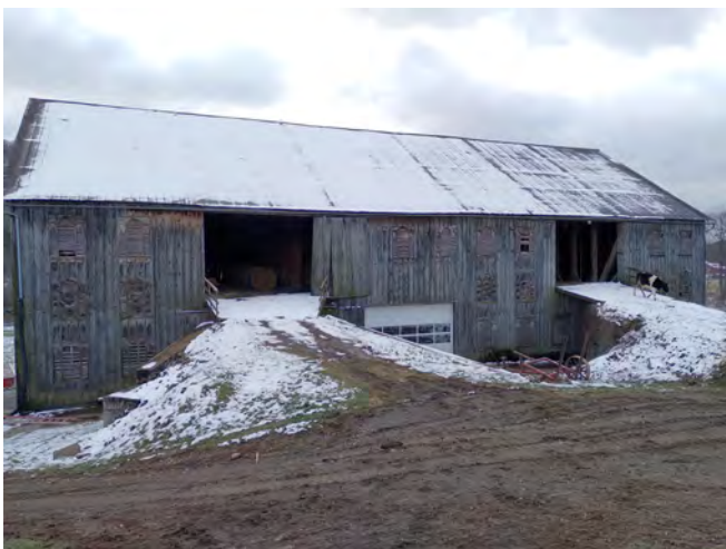
Missing doors and downspout November 17, 2022
