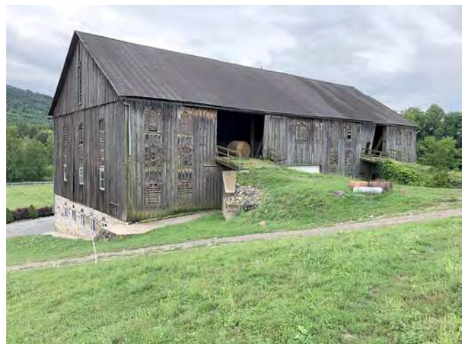
Missing doors, downspout September 21, 2021
