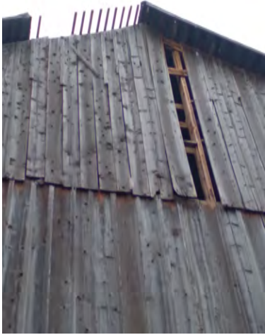
North roof missing (western view) November 16, 2022
