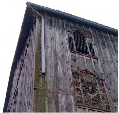
No downspout November 16, 2022
