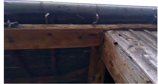
Damaged gutter November 16, 2022
