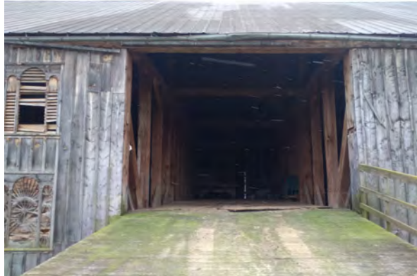
Missing door, damaged gutter, weak roofing November 16, 2022
